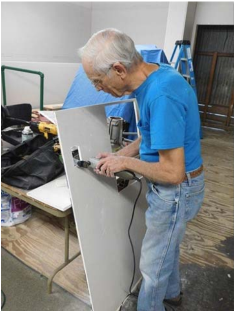
Railroad Museum Curator, Ken Murdock, works on a piece of sheetrock for the new meeting room and museum expansion area.
